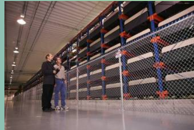
46 MW battery storage
